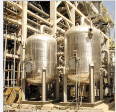
TUPRAS AIR DRYER
