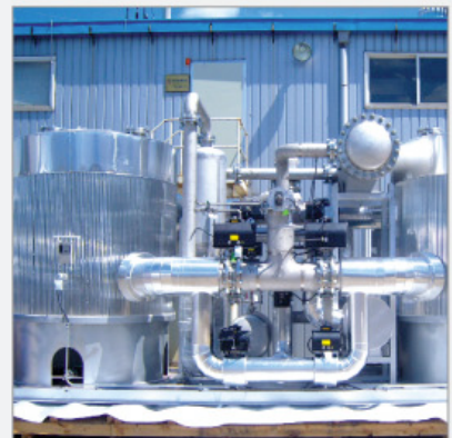
SK CHEMICAL N 2 DRYER
