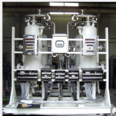
RAS LAFFAN AIR DRYER
