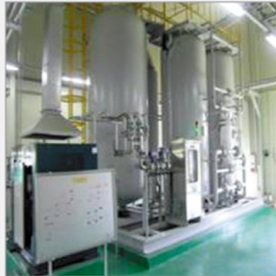
LG INNOTECH N 2 GENERATOR
